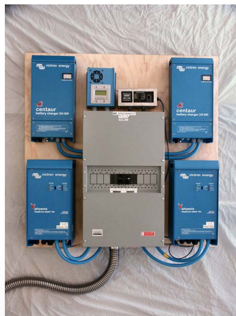
Mega Victron Power Board
